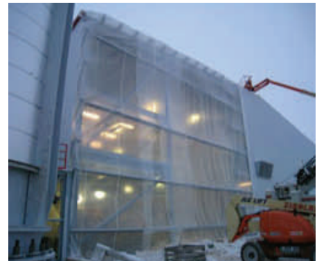
12/18/2008—Energy Center awaiting boiler delivery by rail
